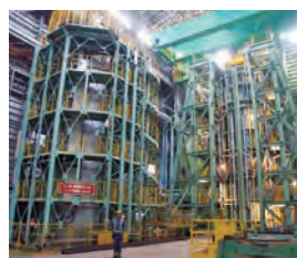
熱処理炉 Heat Treatment Furnace
