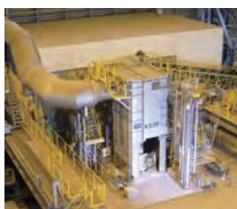
取鍋精錬炉 Ladle Refining Furnace
